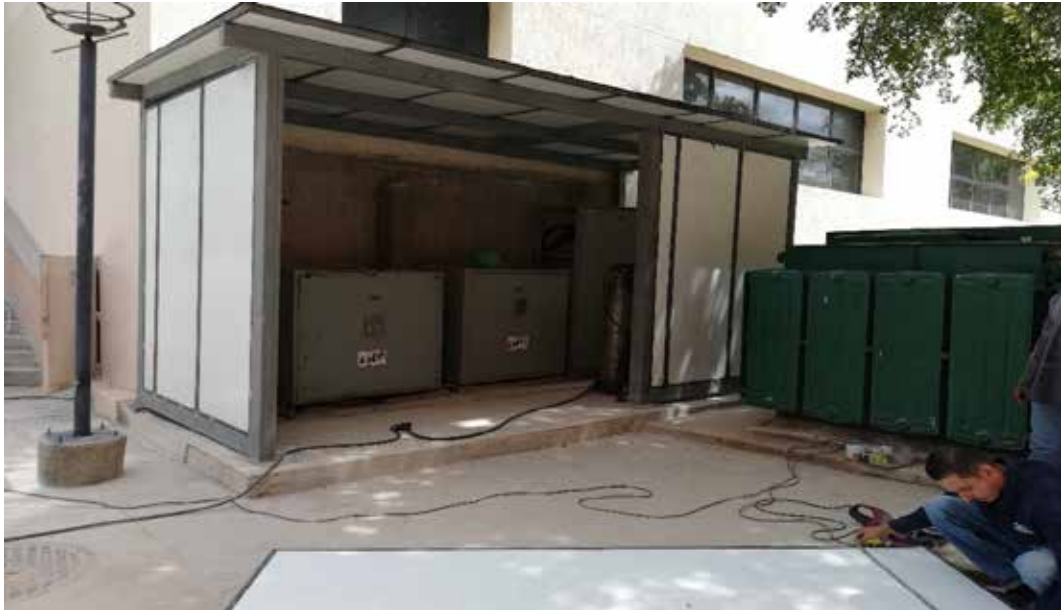
Figura 42 – Transformadores secos y Pad Mounted
