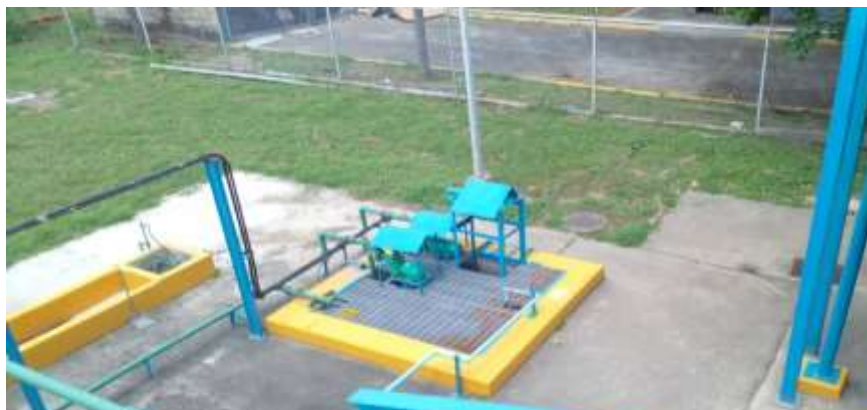
Figura 10. Tanquilla T – 06. Tanque principal
