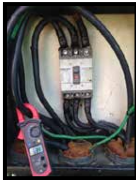
Figura 23: Breaker Principal AC
