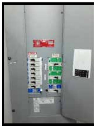
Figura 28: Tablero Principal AC y DC
