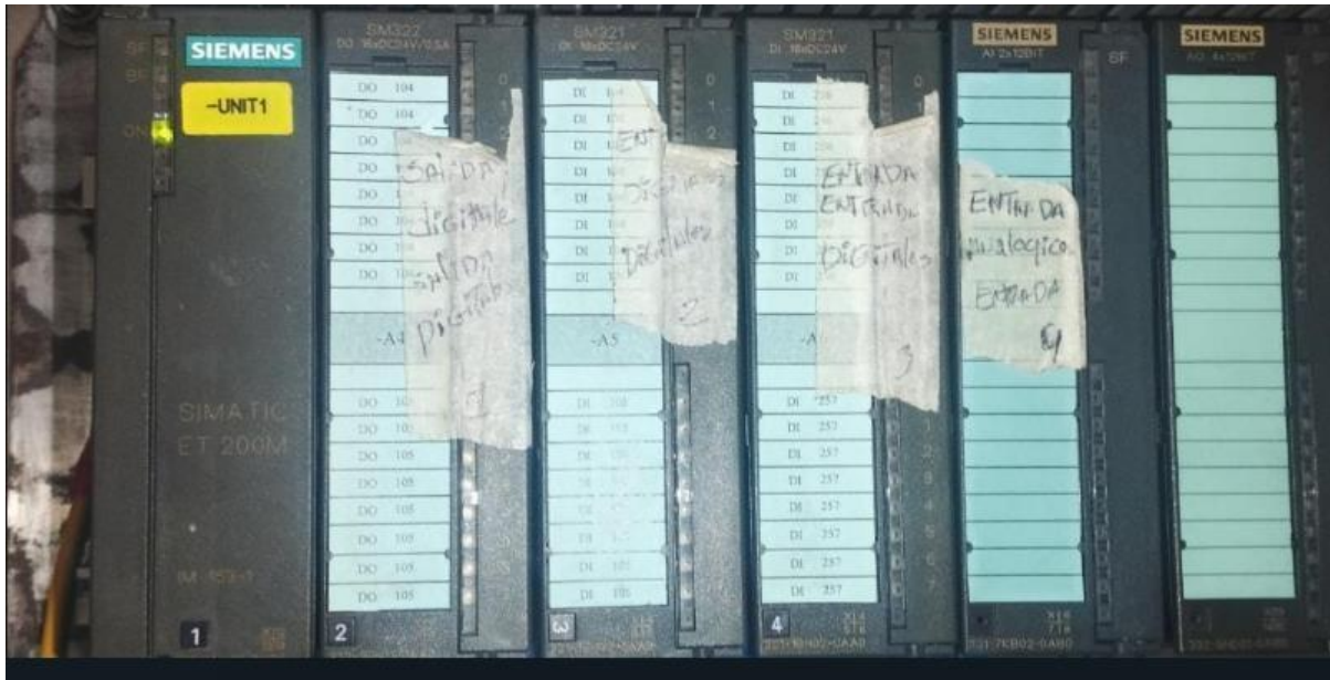
Figura 32 PLC SIMATIC ET 200M
