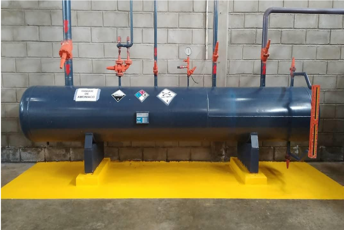
Figura 10: Tanque colector de Amoniaco
